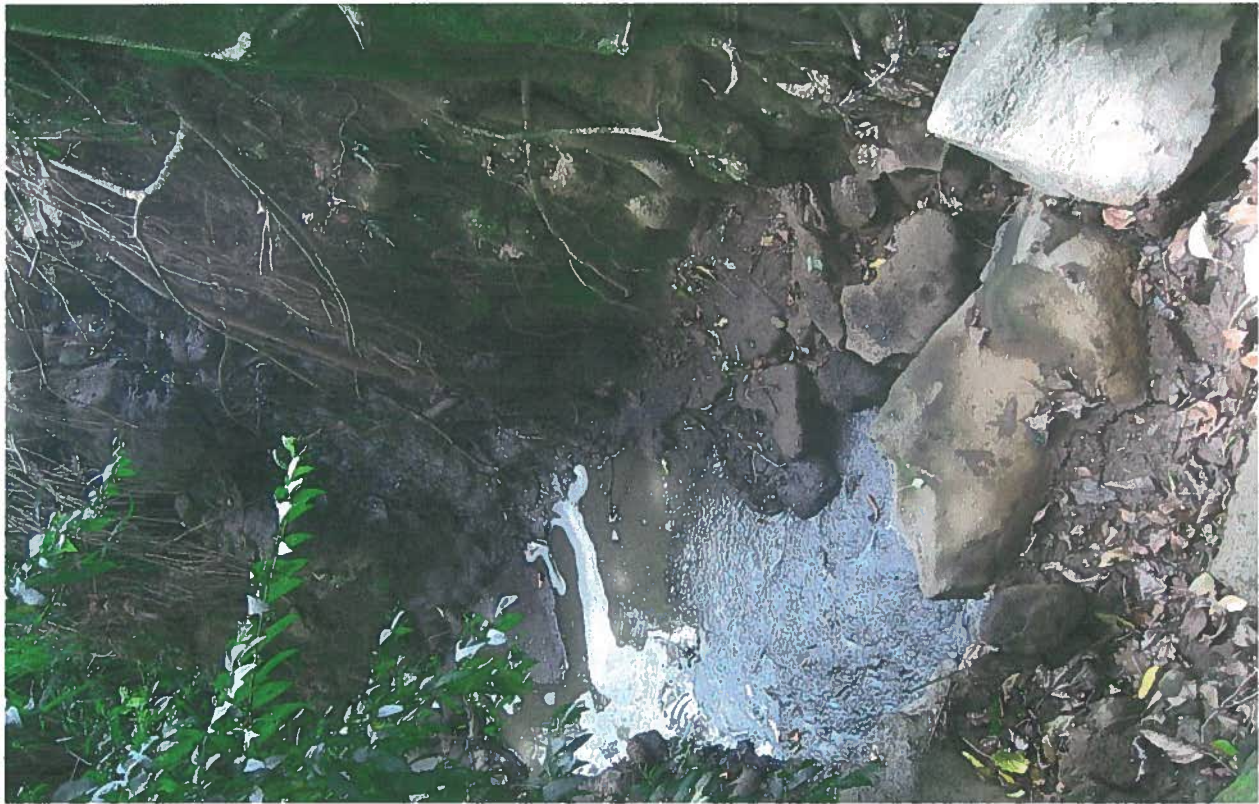
Photograph#14- This is another photo of the brown sewage water in the stream, with the sewage water entering from the left side of the photo and continuing to flow downstream toward the left .
