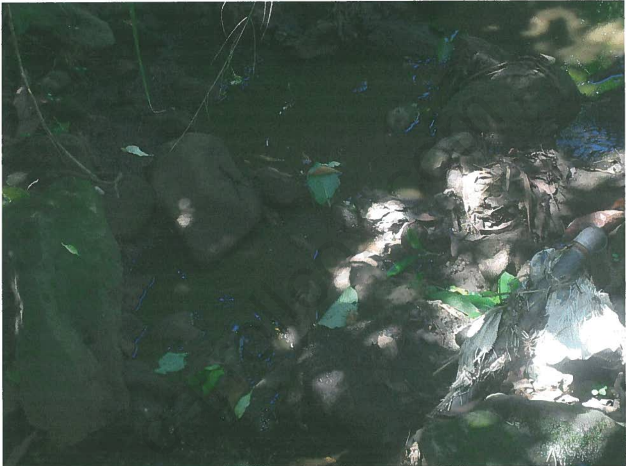
Photograph#1-This is a photo of the brown turbid smelly water flowing in the stream in the Ookala town and residential area where the complaint originated from.
