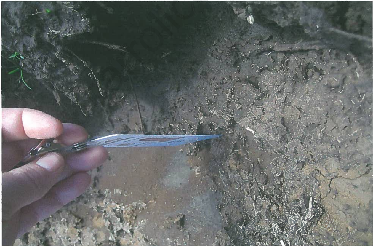
Photograph#17- This is a photo showing the depth of the erosion channel.
